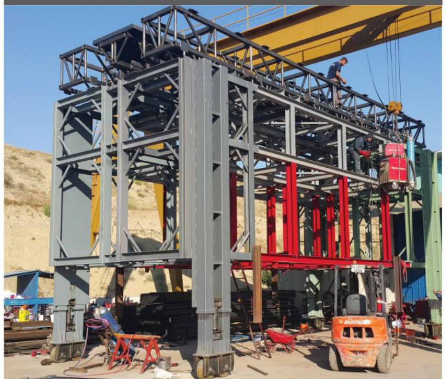
Tunnels for High Speed Train systems in Ankara, Turkey- 3 specially designed hydraulic cut and cover type infrastructure tunnel form work units used to lay 3kms of tunnels.
