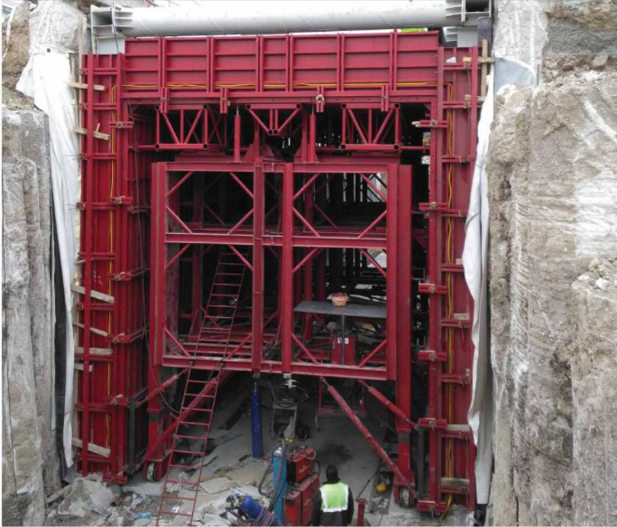
HIGH SPEED TRAIN TUNNELS, Ankara, Turkey 3 mega tunnelling formworks specially manufactured 8m high x 7m wide x 12.5m utilized to cast 3kms of high speed train line in Ankara, Turkey
